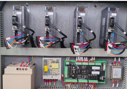
Board control system
